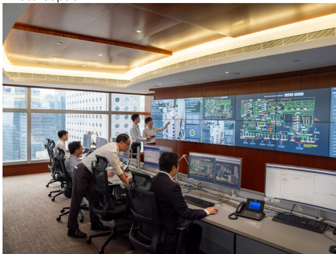
Hongkong Land's Centralized Monitoring Centre (CMC) in Exchange Square
